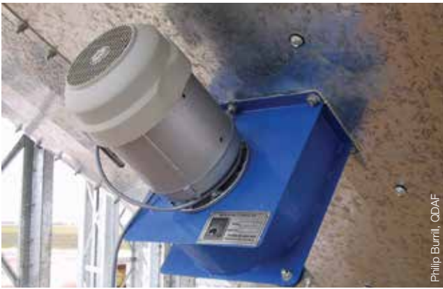
Aeration fans fitted to silos can rapidly reduce grain temperatures.
